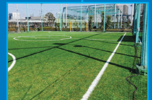
Construction of Futsal Court Location: Behind Blk 41 Teban Gardens Road Estimated Completion: 2nd Quarter 2022
