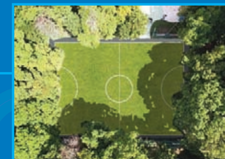
Construction of Futsal Court Location: In front of Blk 410 Pandan Gardens Estimated Completion: 2nd Quarter 2022
